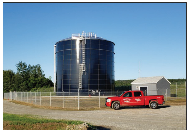
View of the new 1 million gallon glassed-to-steel water storage tank at the Hooksett Village Water Precinct.
